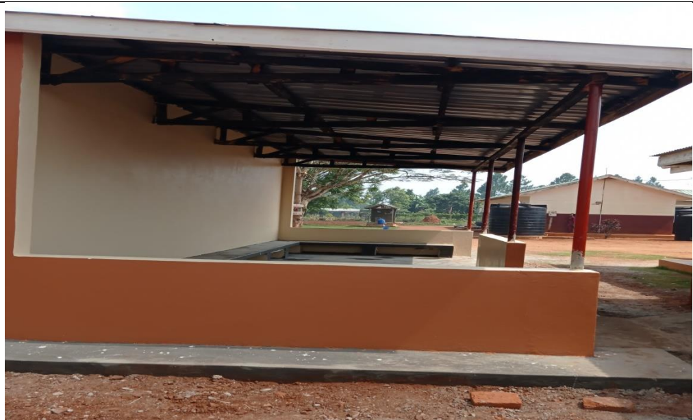
Construction of a waiting shade at OPD at Mbulamuti HC III Mbulamuti Sub county DDEG/EU funds
