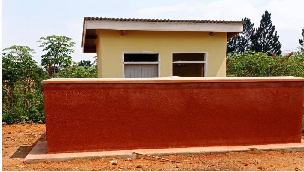
Construction of a two stance pit latrine at Butansi HC III in Butansi Sub county DDEG/EU funds
