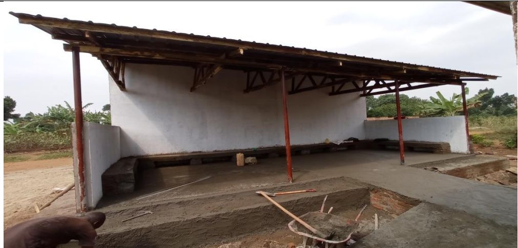
Construction of a waiting shade at OPD at Bubago HC II Kisozi Sub county DDEG/EU funds
