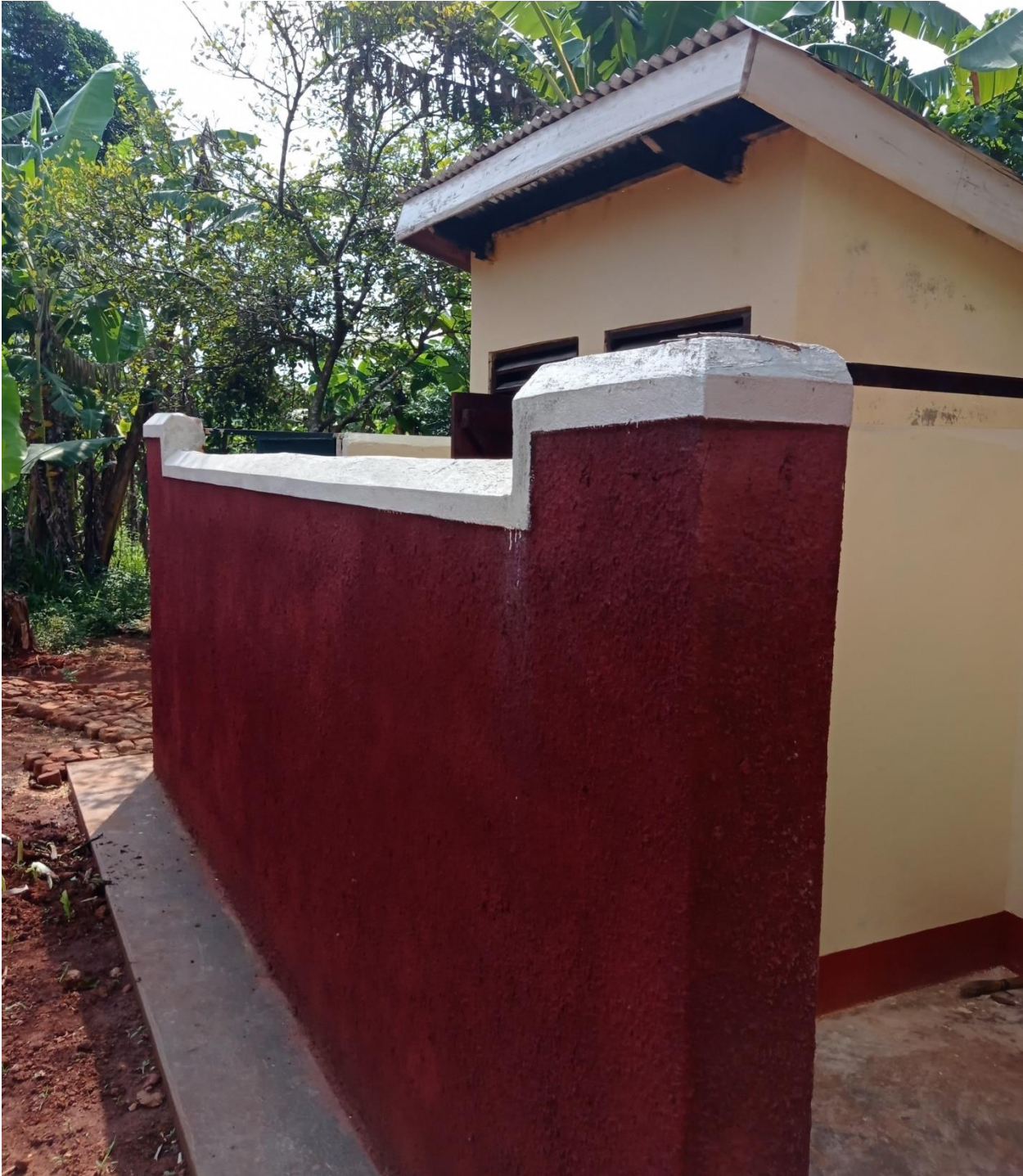
A 2 STANCE PIT LATRINE FOR THE TEACHERS' HOUSE AT KASAKA P/S IN BULOPA SUBCOUNTY
